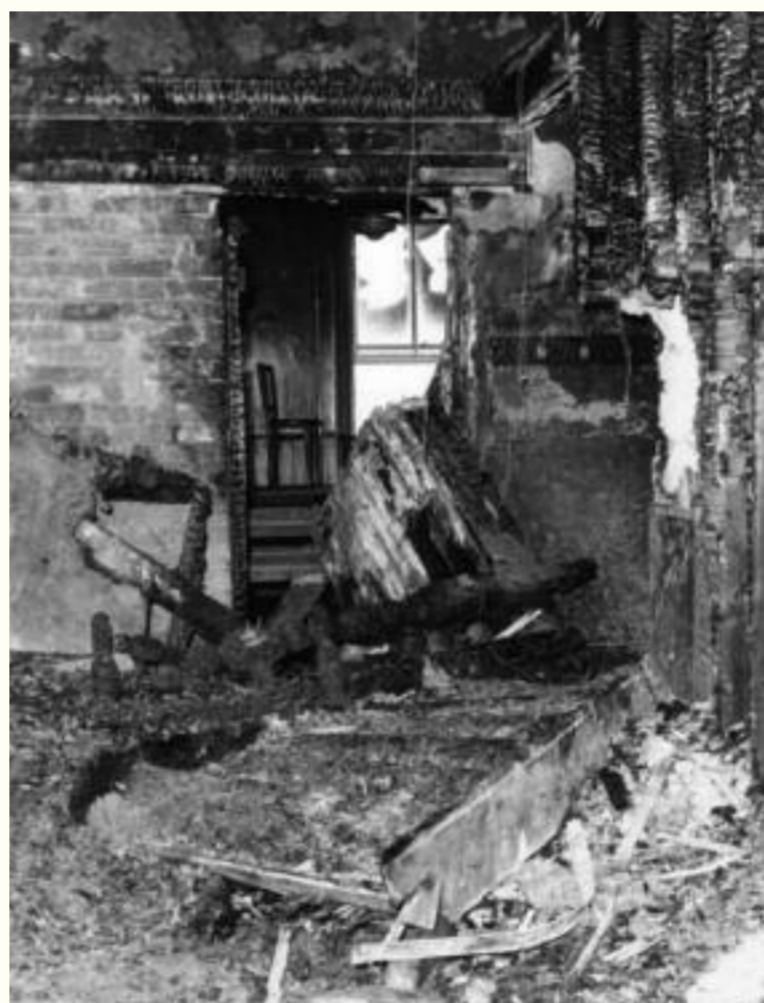
The fire blackened remains of the old attic west of the Tower after the fire of 1954. Note the chair in the background.
